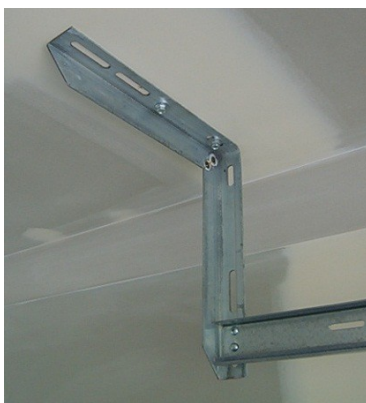
Figure 5 – Typical Rear Track Hangers for End of 2400 Horizontal Track (old style angle Roller Door bracket shown)
